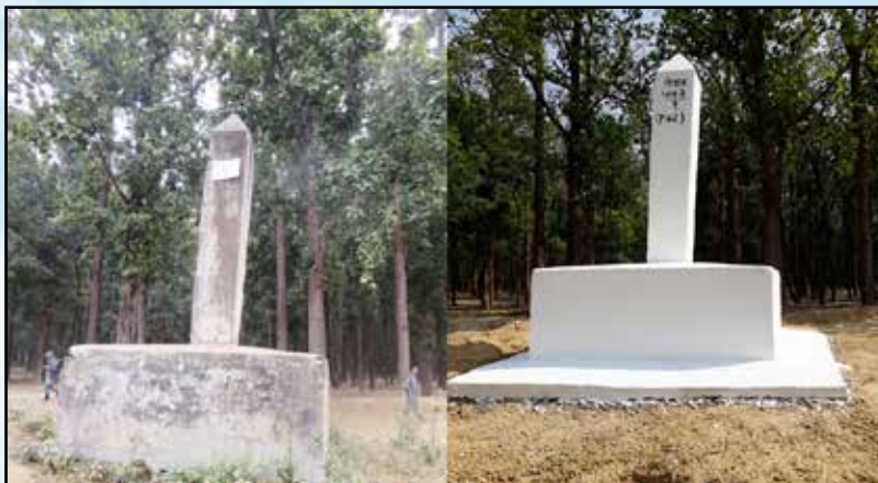
The Nepal-India Joint Field Teams conducting joint field works in Nepal-India border area. Among different tasks performed by Field Teams we can see the same boundary pillar before and after repair works.
